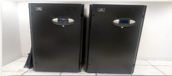
Energy Efficient Equipment's
